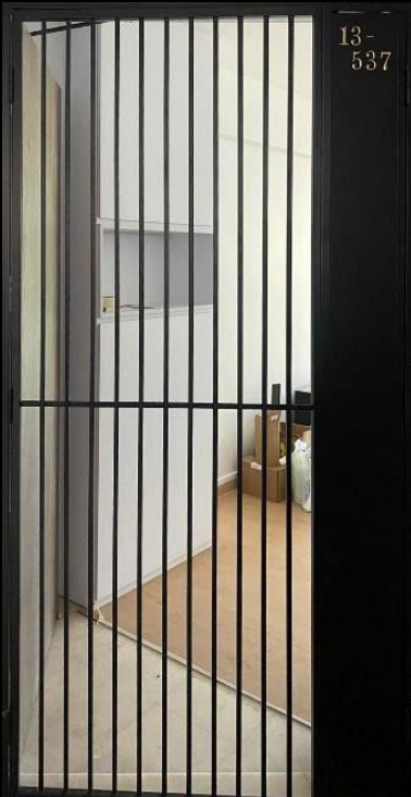
Gate design with side plate not flushed
